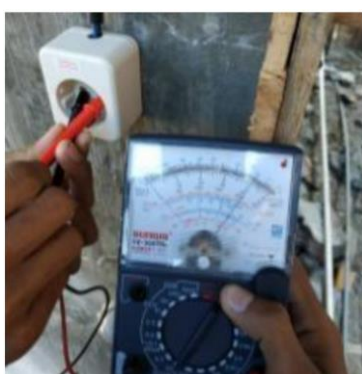
Gambar 4. Uji Coba tegangan output panel surya
